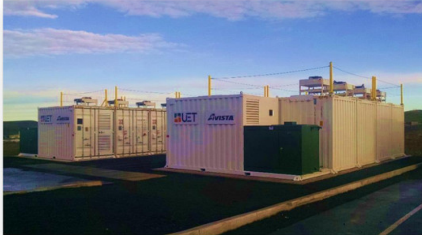
Photo: Pullman Energy Storage Project
